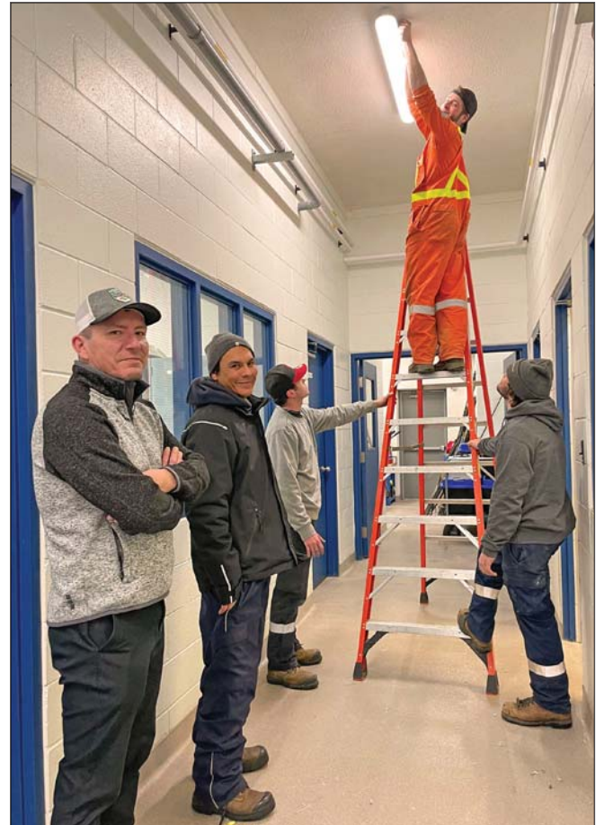
The Water Treatment Plant got an Energy Efficient Facelift through Save On Energy's First Nation Community Building Retrofit Program! Pictured here are IES Manager, Richard Shawanda, Community Energy Champion, Ryan McGregor and the talented gentlemen of Steel Control Services. Shawanosowe School and WRFN Administration will also be receiving upgrades. Nishin!
