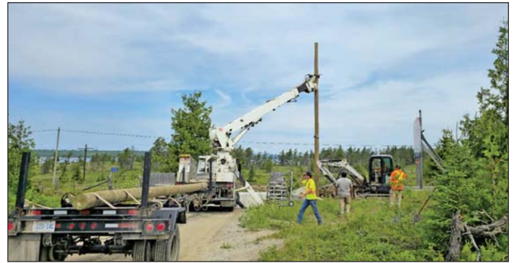
☀️ A new solar-powered street light was installed by Hwy 6 & Sunshine Alley Rd. to provide efficient, eco-friendly lighting using the power of the sun.
